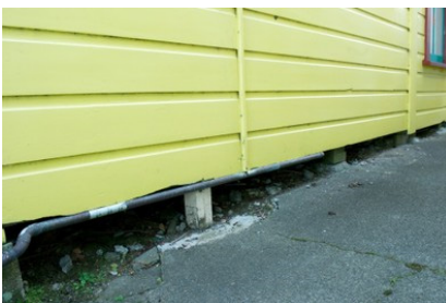
Figure 1: Areas of subfloor space with insufficient clearance
