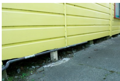
Figure 7: Areas of subfloor space with insufficient clearance
