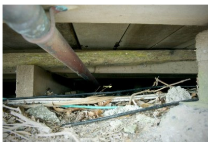
Figure 8: Areas of subfloor space with insufficient clearance
