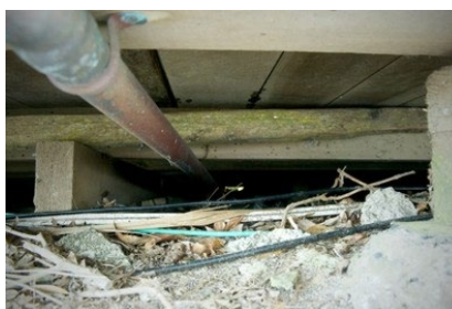
Figure 8: Areas of subfloor space with insufficient clearance
