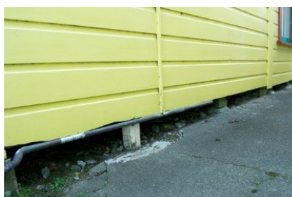
Figure 7: Areas of subfloor space with insufficient clearance
